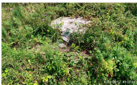
2024-08-12 Collapsed well house & sweep over Well Sweep at Well Sweep Lane & Kings Highway.
